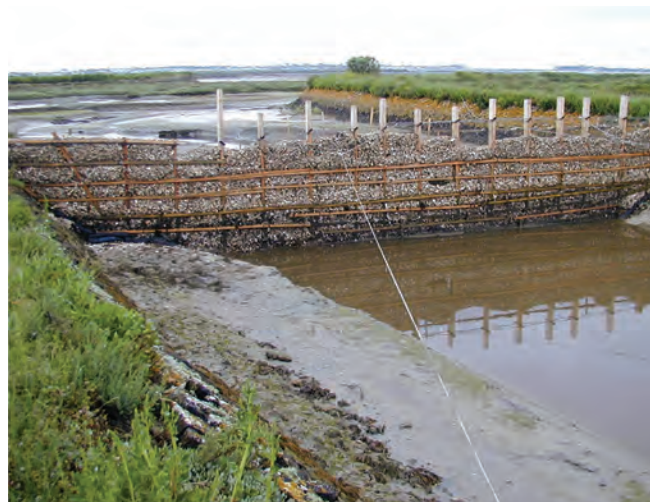
▲ Figure 21: Barrier constructed from oyster-shells, held in place by stakes and nets.
